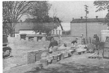
Bricklayers work on the walls of the new Aurora Town Public Library at Main Street and Whaley Avenue in the summer of 1963.
